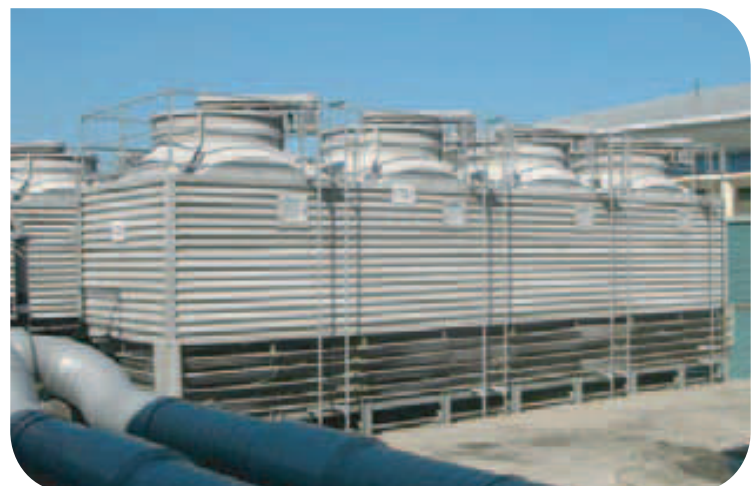
:: SG Buloh Hospital, 3000 HRT.
